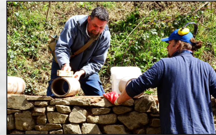
Matt supervising the building of the Kingfisher Wall in 2016 Photo: Lexi New
